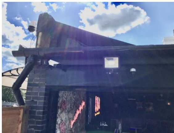
Photograph 5: view of upper side façade construction as seen from rear of 74 Oxford Road
